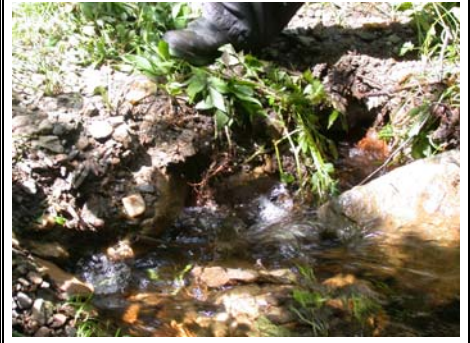
Pt 9: ponceau amont obstrué
